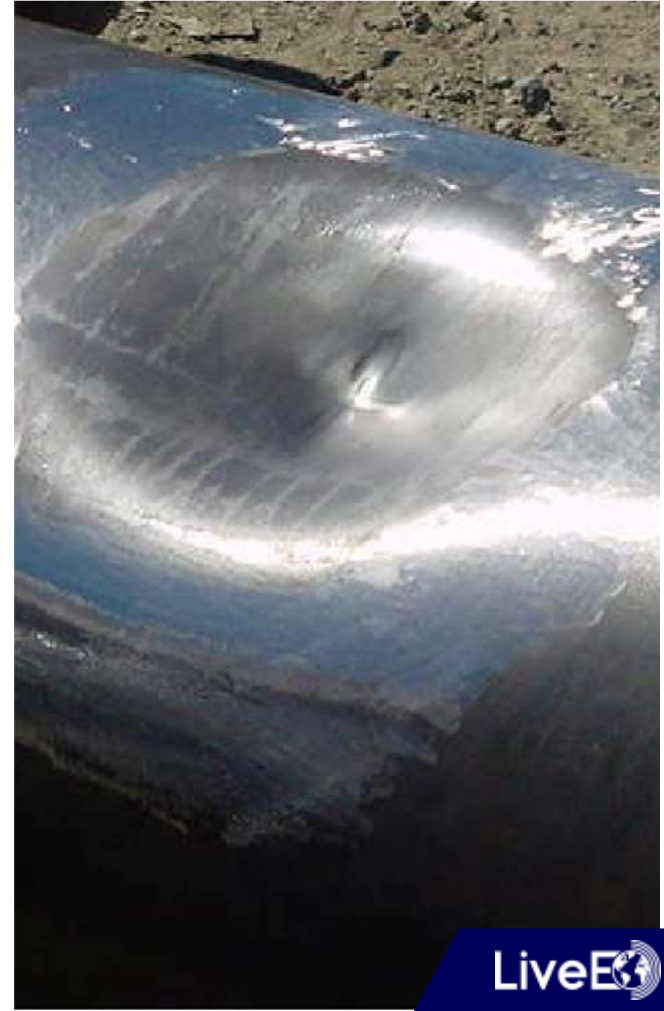
Stressed wall of the underground steel gas pipeline
