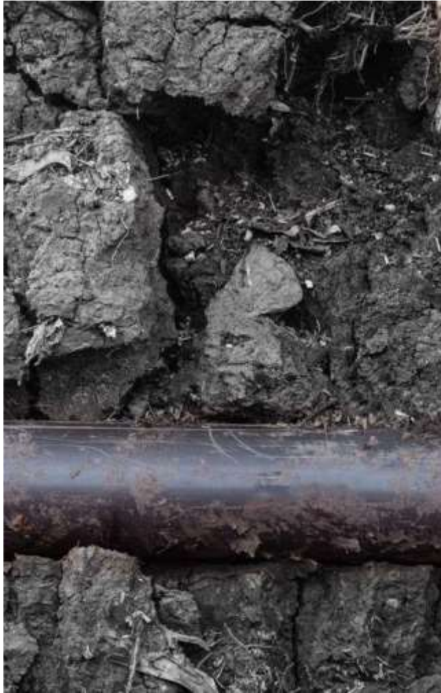
Underground steel gas pipeline
