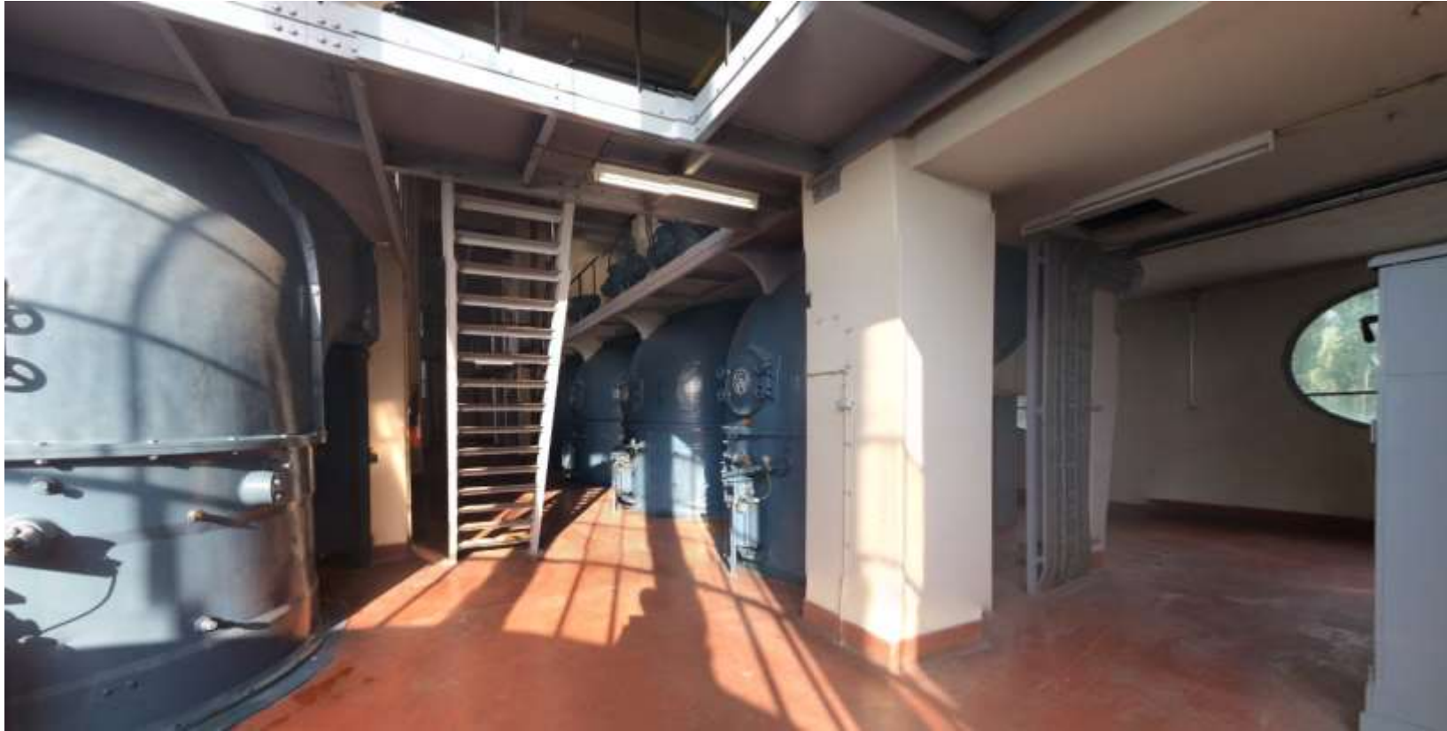
Inside one of the ventilation buildings of the Maastunnel, Rotterdam: 1942 - ...
