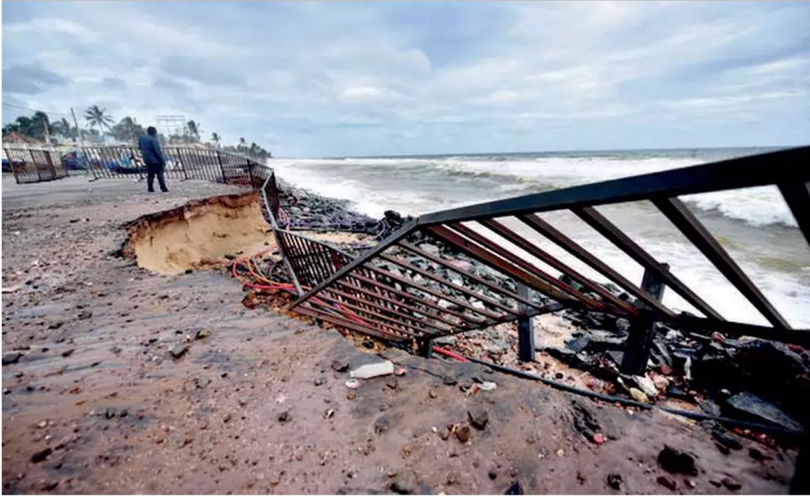
Road destroyed due to coastal erosion(Times of India,2021)
