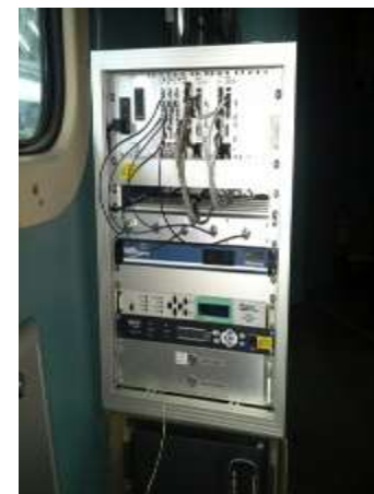
Rack Inside the train
